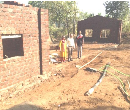
Visit of Dr. Prashant Kambale , Assistant commissioner, Mini polyclinic tal. Badalapur and Dr. Smita Jinturkar, Livestock development officer (Extension) for Verifying Poultry Shed Construction Work
